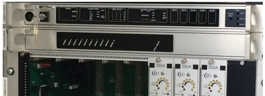
Photo shows from the top: ZX100 PAGA system processor, underneath this is the LTD002X expansion status display unit.
