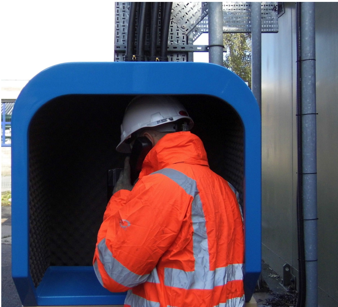
PP-W-03 Page / Party station installed in an AH23 acoustic hood
