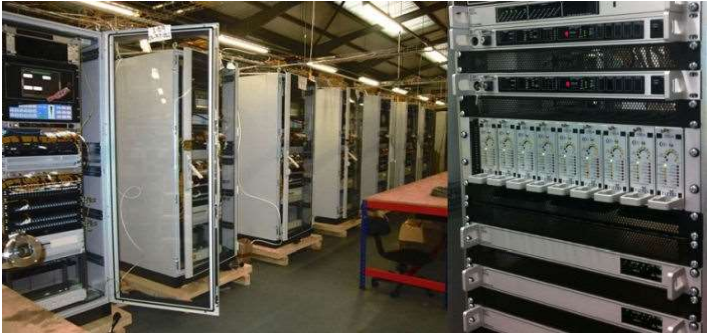
Networked multi sector PAGA system pictured during in house testing – a distributed approach is specified for large sites to improve efficiency and integrity.
