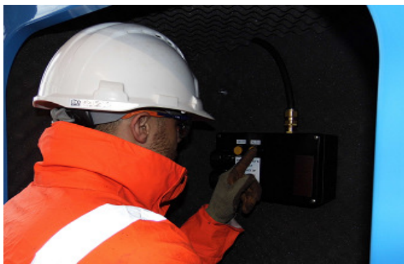
Photo shows AP10-02 in an AH23 Zitel acoustic hood
